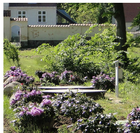
Mars 3000 installed at Boarding School
